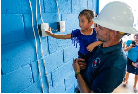
After spending three weeks at the project site, the lights finally came on for village residents on Tuesday, September 13. The project consisted of building power lines and wiring 84 structures, including one elementary school and two churches.
