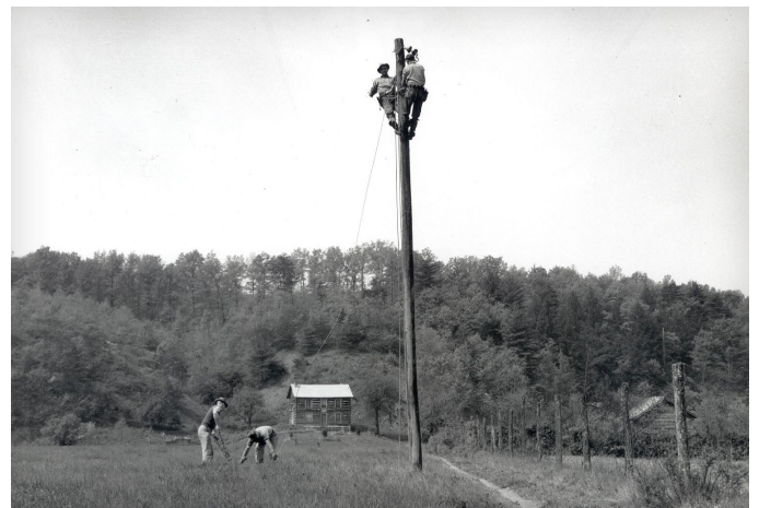
Linemen work to bring life-changing electric service to rural areas in the early 1940s. Reprinted with permission. @National Rural Electric Cooperative Association.
