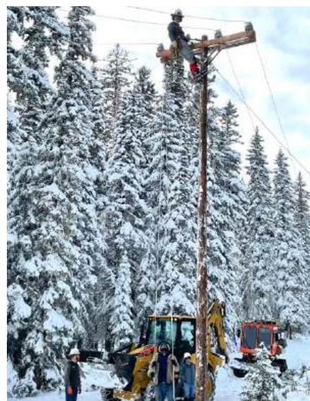
La Plata Electric crews work to restore power to members in the Durango area during a recent snowstorm. Photo courtesy LPEA.
