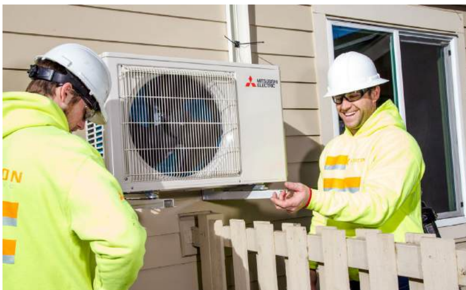
The condenser for a mini-split is often mounted on an exterior wall. Photo by Marcela Gara, Resource Media.
