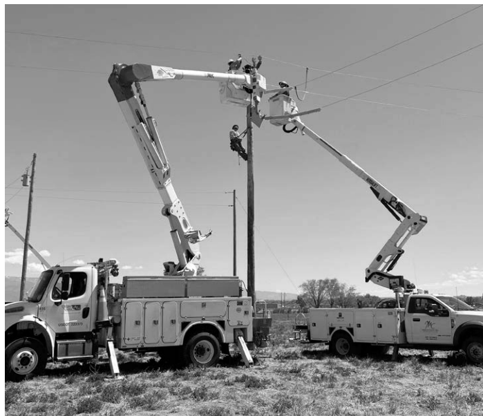
MCREA lineman Andron Brown (on pole) instructs two students changing out a fused cutout at Mesa Hotline School.
