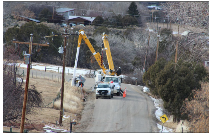
▲ An EEA linecrew upgrades a distribution line on Road T.5 earlier this year.
