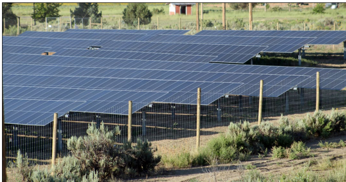
▲ Totten Lake solar generation station located northeast of Cortez is one of three local renewable generators that delivers clean energy to EEA members.
