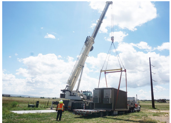
▲ Cement-walled fiber huts provide secure housing for network connectivity components and serve as the "nerve centers" of fiber-to-the-home distribution networks. To date, five huts have been delivered and installed to support MVEA's growing fiber network.
