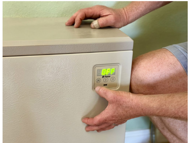
▲ Brad adjusts the new electric thermal storage (ETS) heater at the couple's home. SIEA helped facilitate the large-scale overhaul of their home to update the home's energy system to electric.
