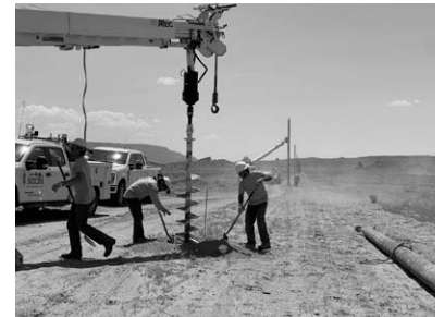
▲ The SDCEA crew works with the Navajo Tribal Utility Authority on the electrification project.
