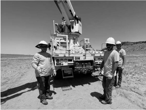
SDCEA linecrew members Caden Creamer, Josh Saar and Colton Blankenbeckler work to bring power to families living on Navajo Nation.
