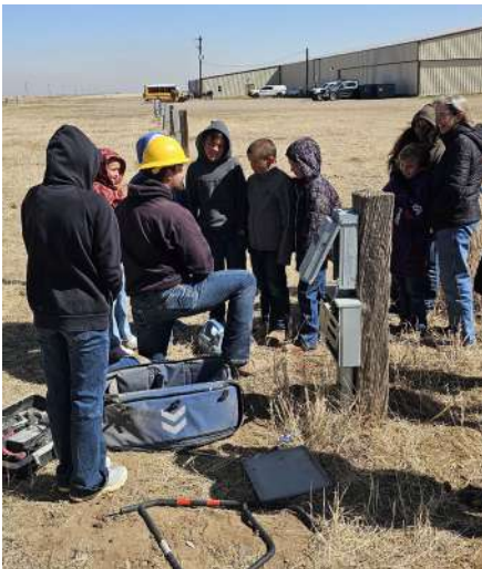
Students attending Youth Conservation Day watch SECPA Journeyman Lineman Trey Redner locate underground power lines.
